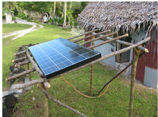
The deployed KYOCERA 135SX solar panel
