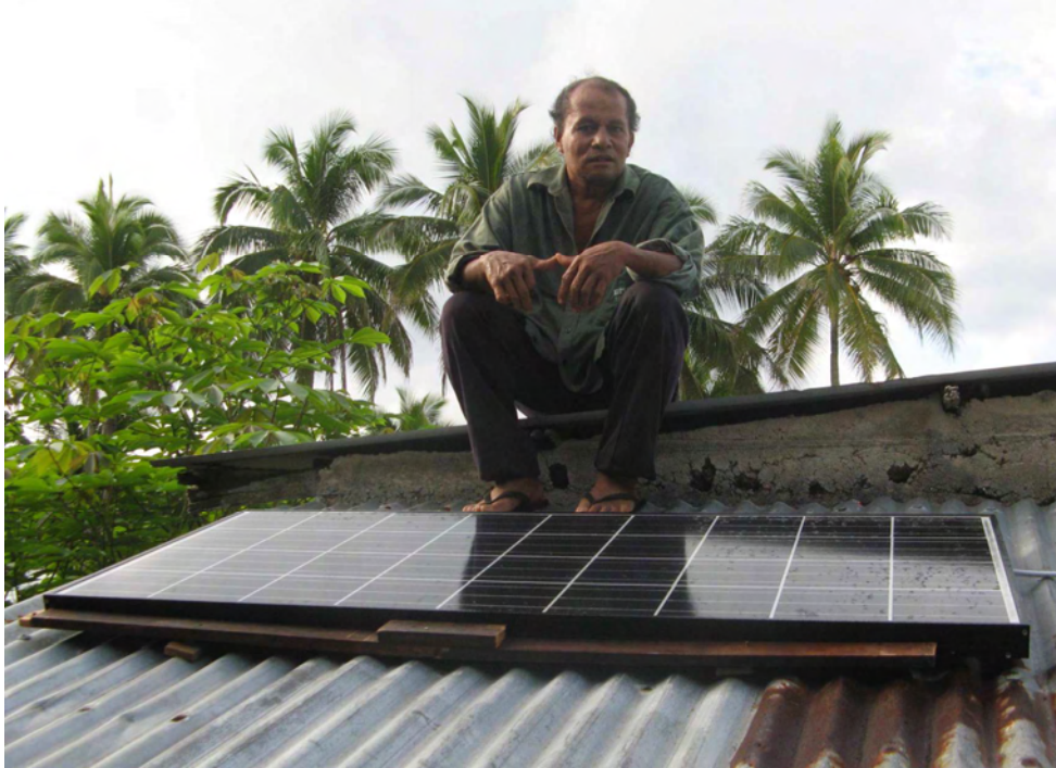
The solar panel was installed on the roof of the main house
